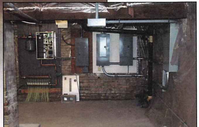
New electrical service.
