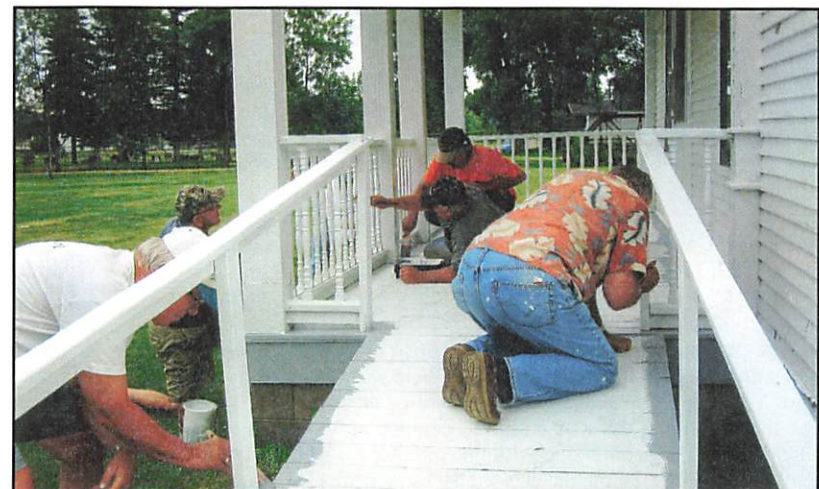
Grafton Lutheran Church men volunteering to paint the back ramp of the Shoultz house.
